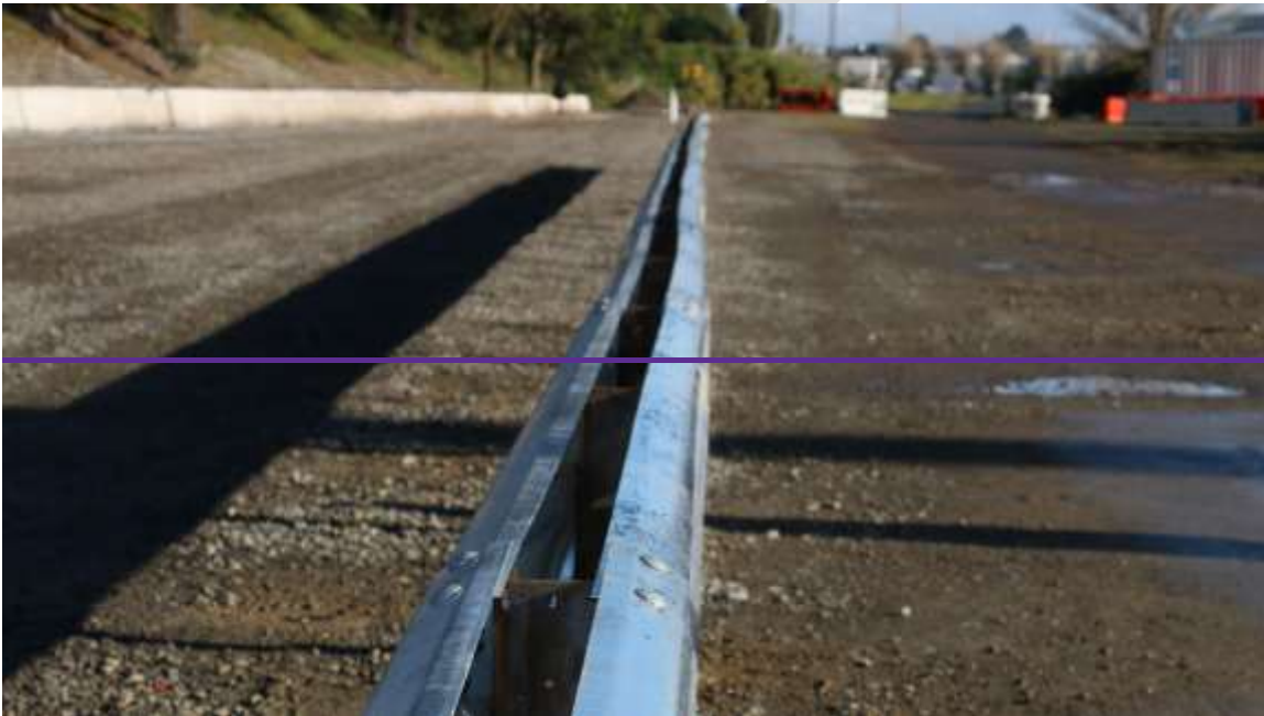
Figure 4-23: ACP Sentry W Beam Median Barrier
