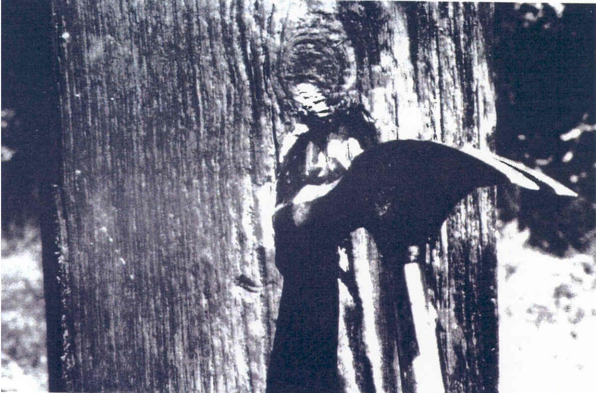
Figure 4.2.3.1 Simple use of a hammer to sound a wood timber. Decay is indicated by a hollow sound.
