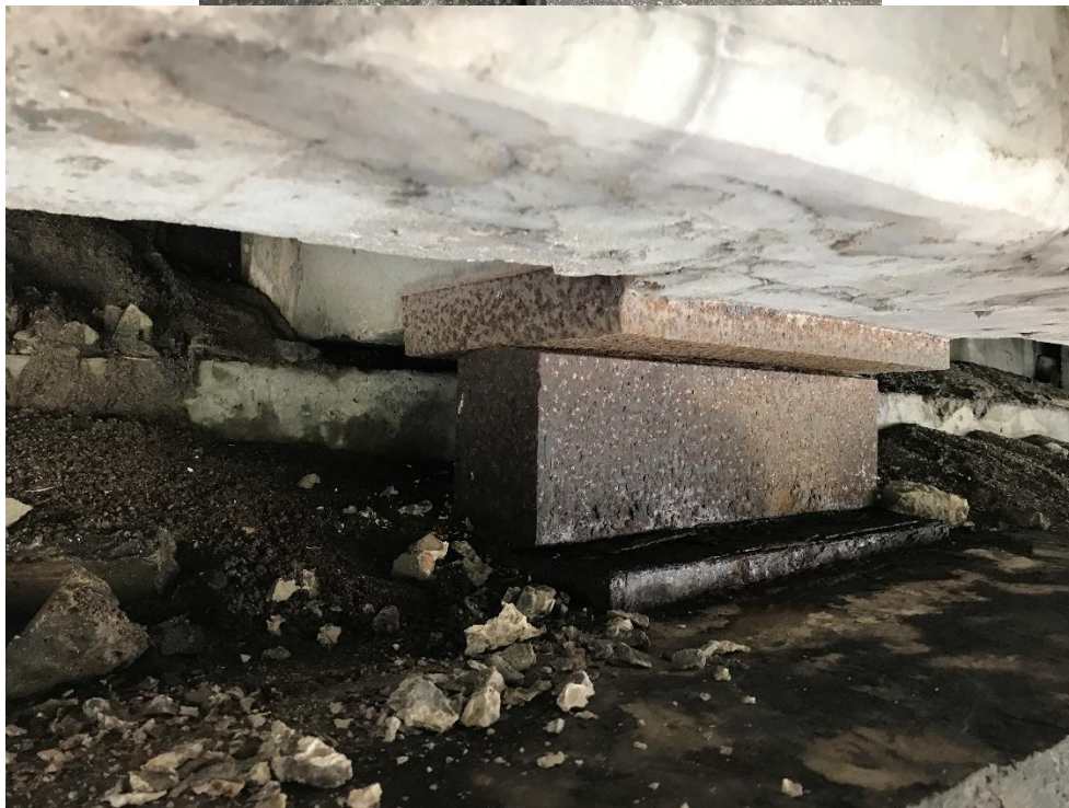
Figure A.11 (c) Paved-Over Joint and Leakage Effects
