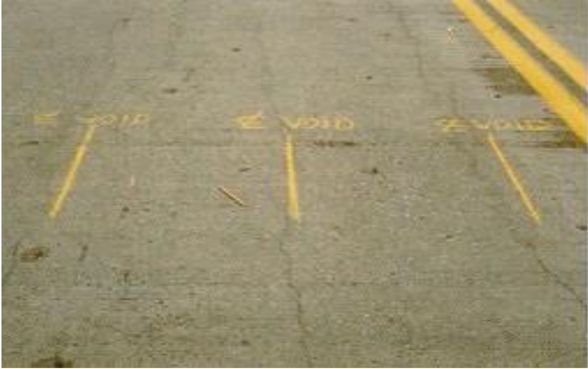
Figure A.8 (a) Exposed Concrete Deck of a Voided Slab
