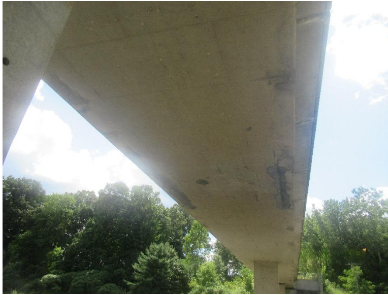
Figure A.8 (h) Thick Slab Soffit
