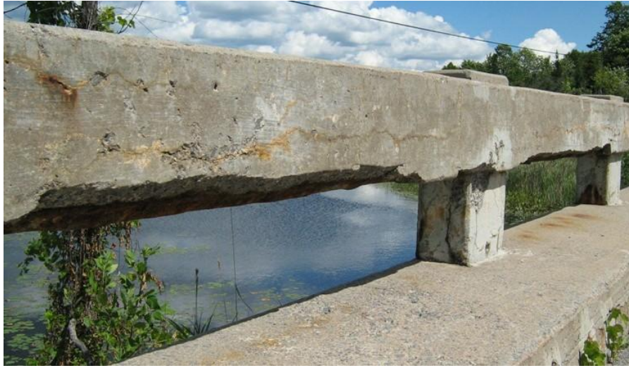
Figure A.3 (g) Concrete Guiderail
