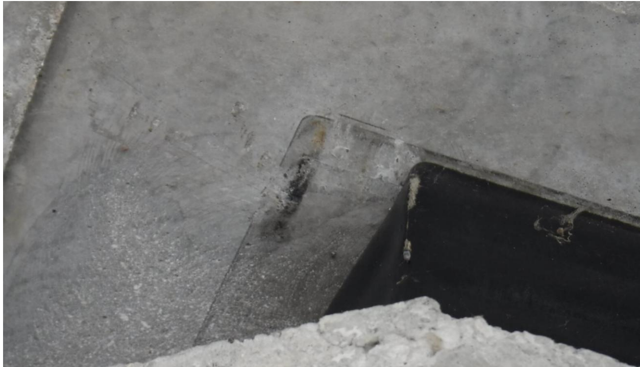
FigureA.1 (h) Abutment Bearing: Looking up at deck soffit and elastomeric bearing
