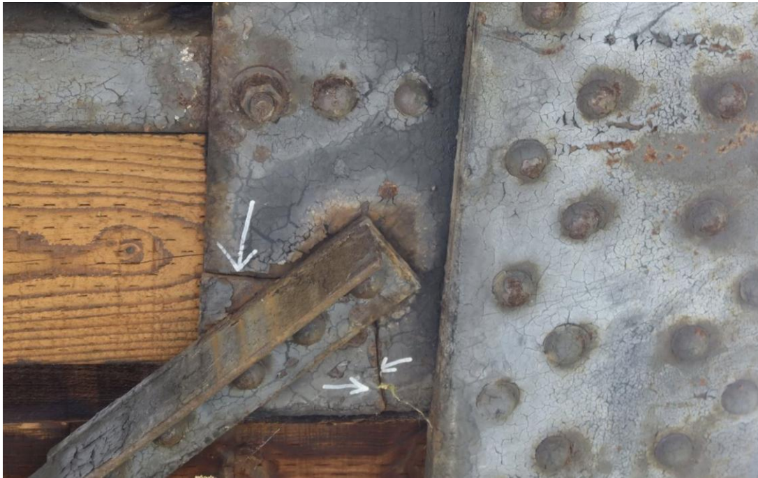
Figure 2.5.6.4 Cracks in Gusset Plate
