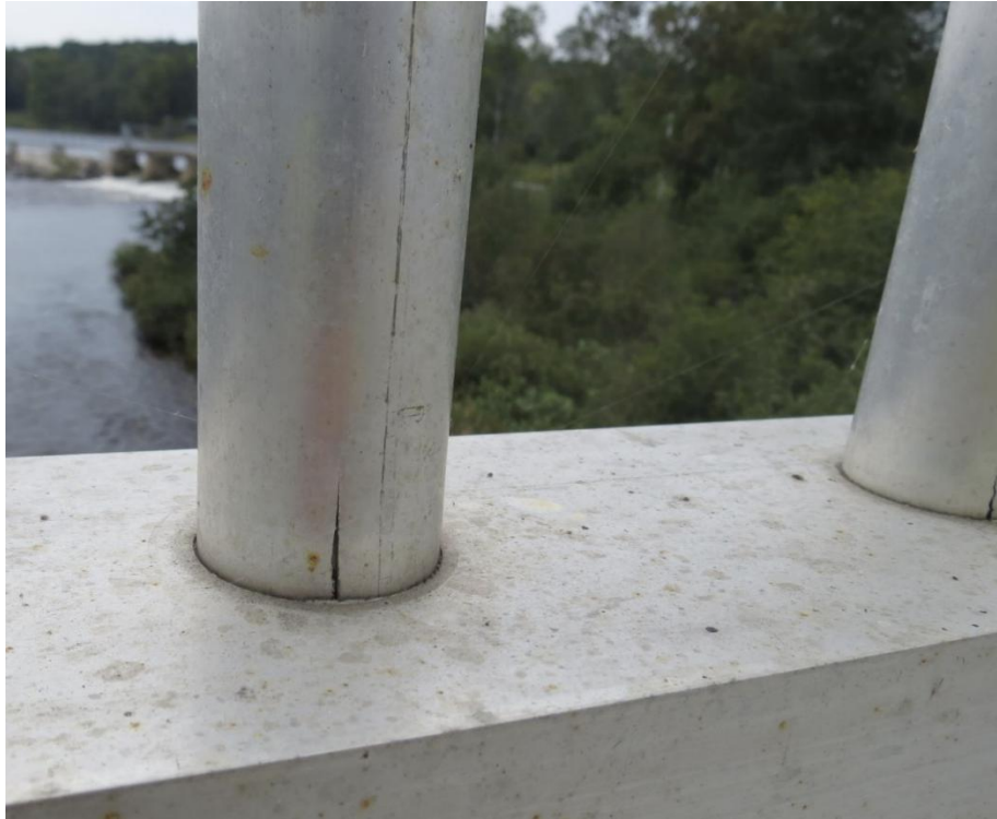
Figure 2.5.7.2 Cracks on an Aluminium Railing
