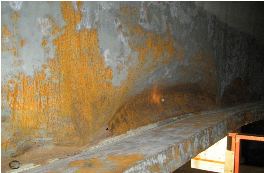
Figure 2.5.6.3 Severe Deformations Caused by Impact
