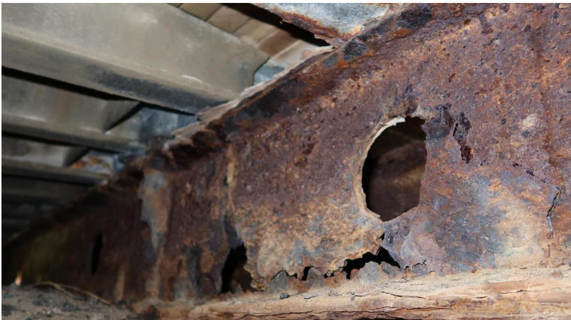
Figure 2.5.6.2 Severe Corrosion of Steel Beam
