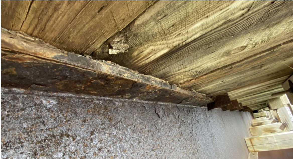
Figure 2.5.6.1 Medium Corrosion of Steel Beam
