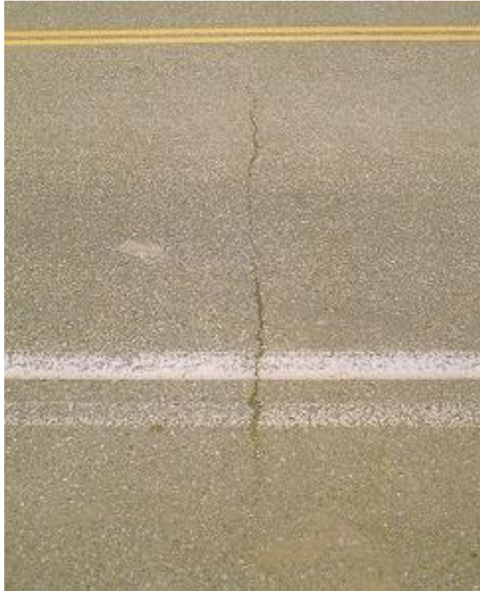
Figure 2.5.8.2 Medium Transverse Crack
