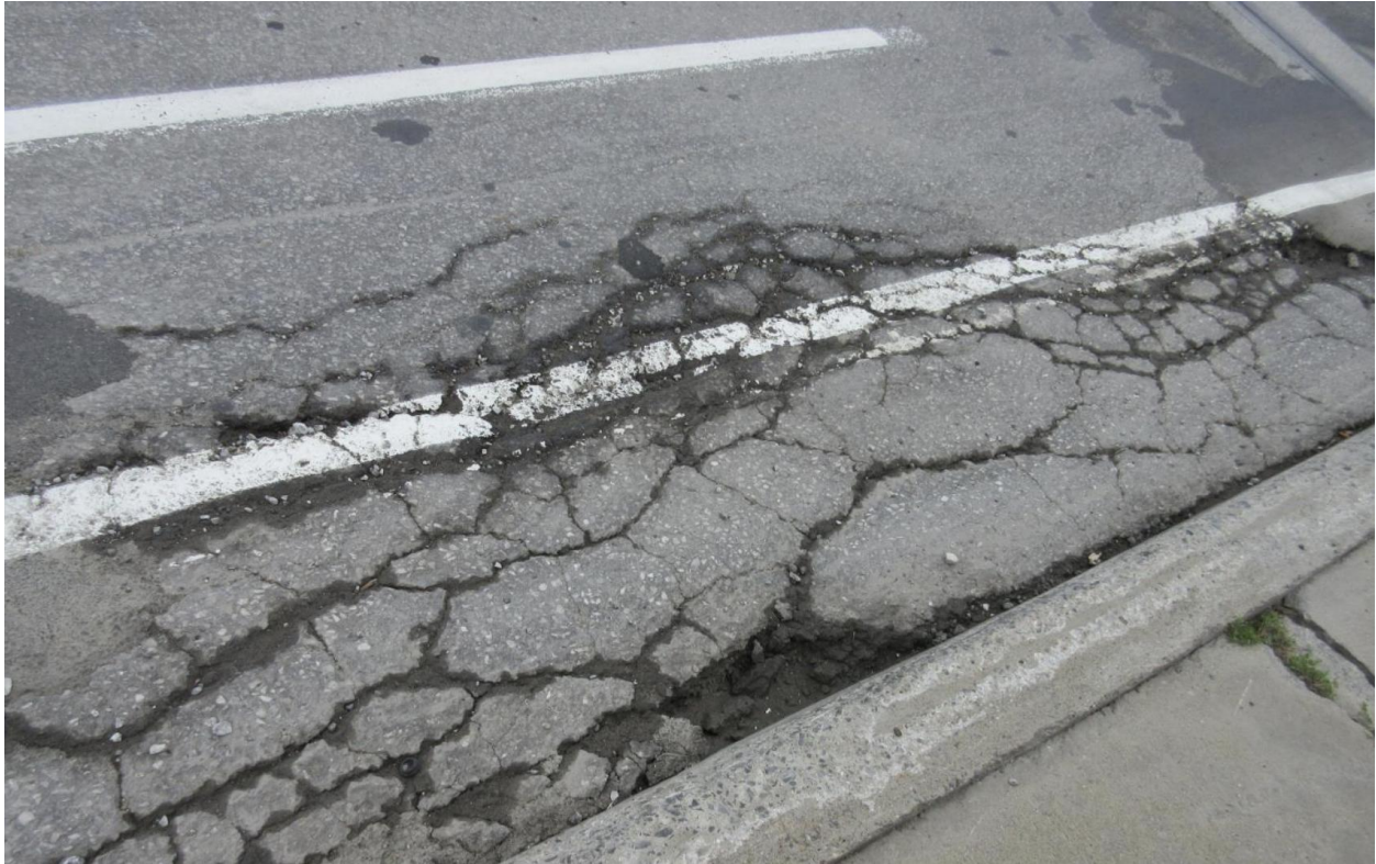
Figure 2.5.8.3 Severe Alligator Cracking
