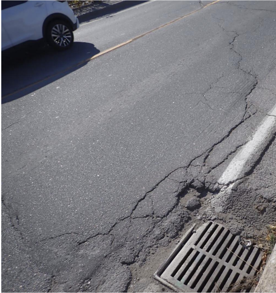
Figure 2.5.8.5 Edge Cracking from Catch Basin
