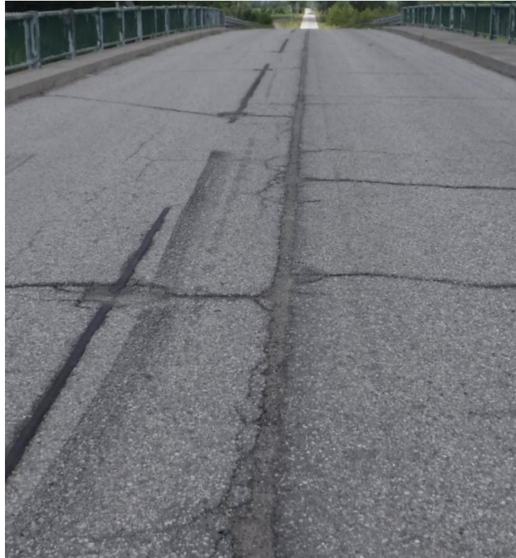
Figure 2.5.8.1 Wide Transverse and Longitudinal Cracks
