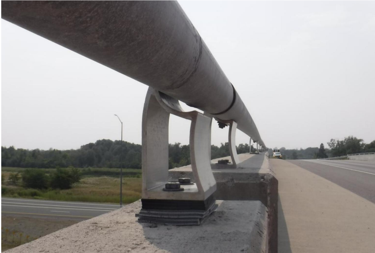
Figure 2.5.7.3 Missing Bolt on Aluminium Hand Railing
