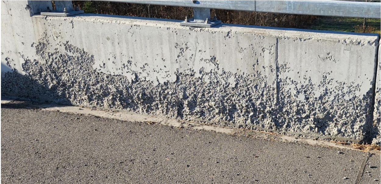
Figure 2.5.4.1 Severe Scaling in a Barrier Wall
