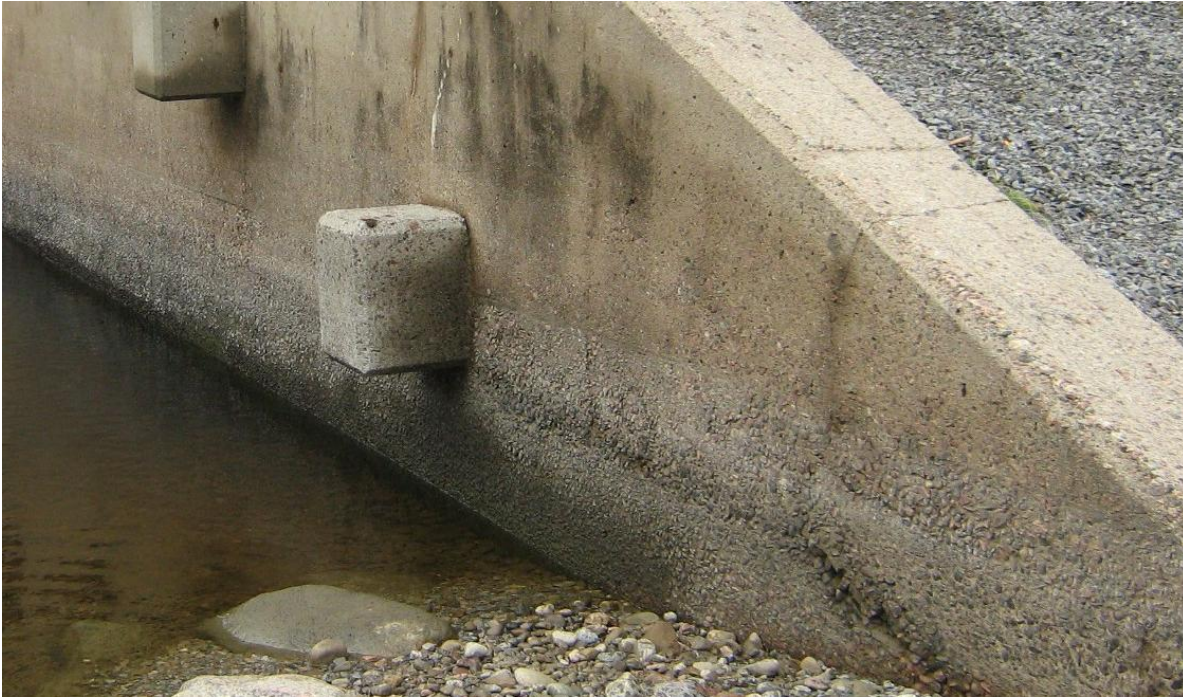
Figure 2.5.4.3 Severe Erosion of a Concrete Wingwall
