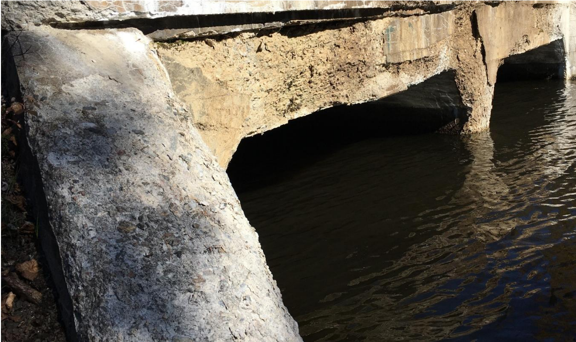
Figure 2.5.4.2 Severe Disintegration of Concrete Culvert
