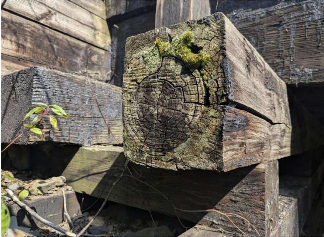
Figure 2.5.15.3 Severe Shakes in Wood Components
