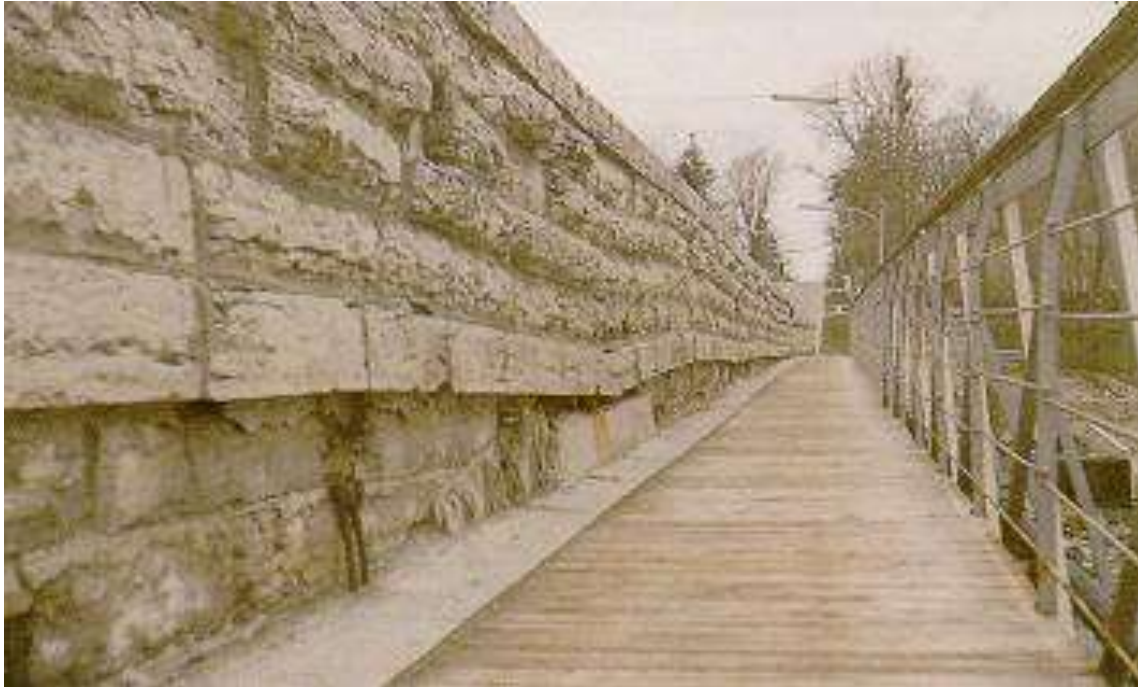
Figure 2.5.14.2 Severe Splitting, Spalling, and Deterioration in Masonry
