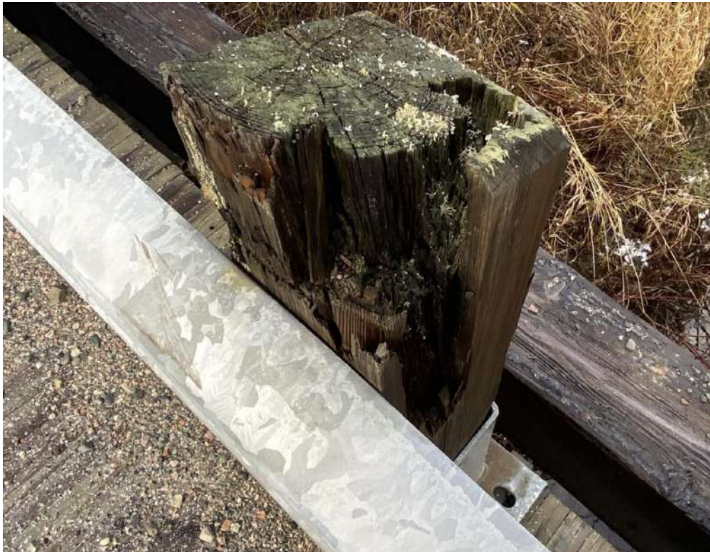
Figure 2.5.15.6 Severe Brown Rot
