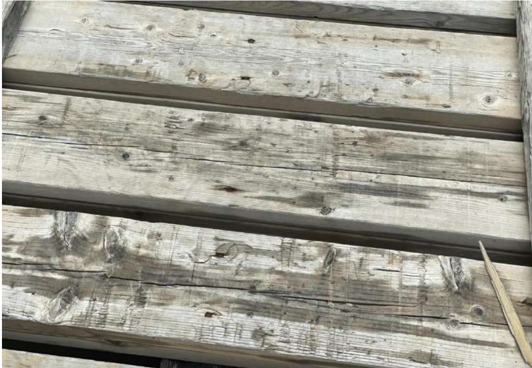
Figure 2.5.15.5 Light Weathering with Medium Checks in Wood Components
