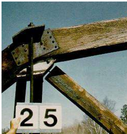
Figure 2.5.15.14 Loose Connection in Wood (25 mm gap measured)
