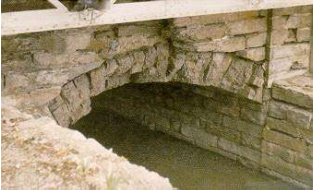
Figure 2.5.14.3 Severe Loss of Mortar and Stone in a Masonry Arch
