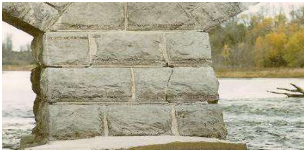
Figure 2.5.14.1 Wide Crack Through the Stone in a Masonry Pier
