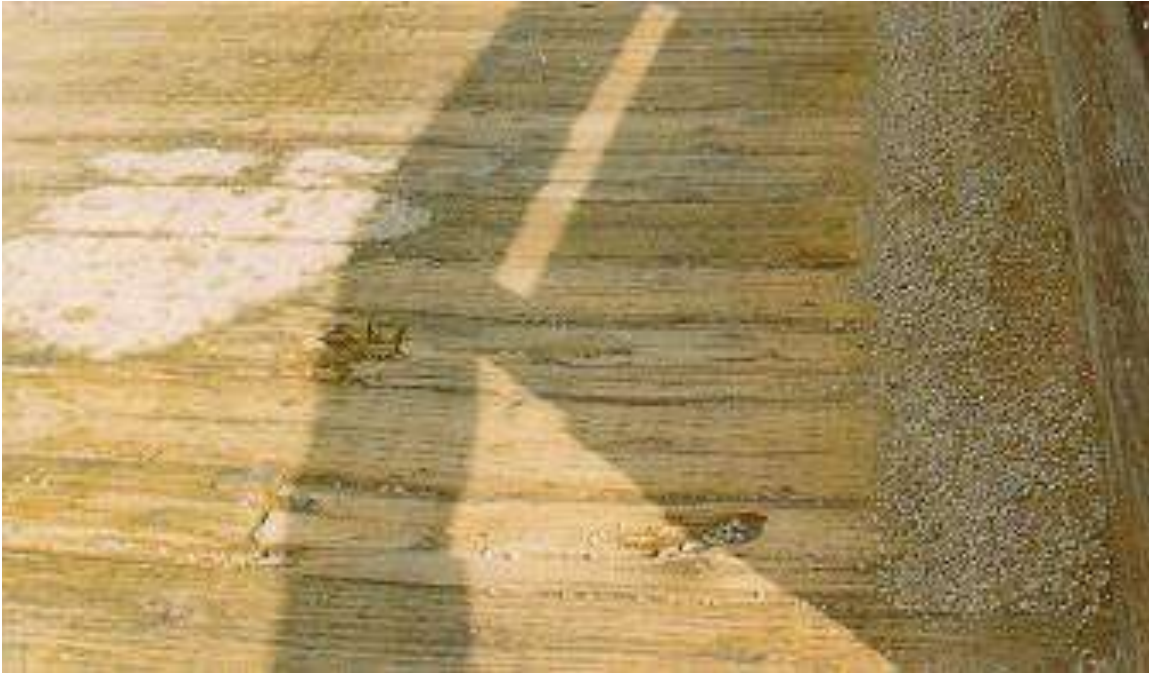
Figure 2.5.15.9 Severe Wear in a Wood Deck
