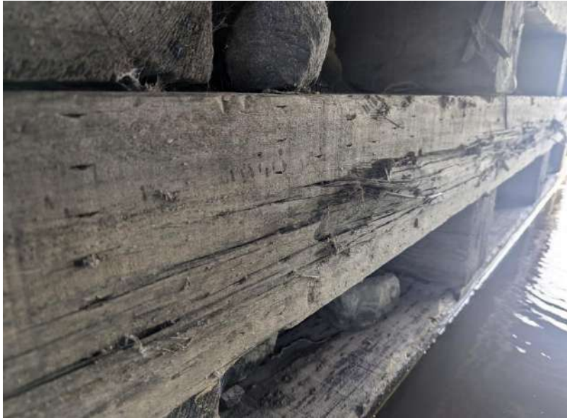
Figure 2.5.15.10 Severe Abrasion and Medium Checking on Wood Crib
