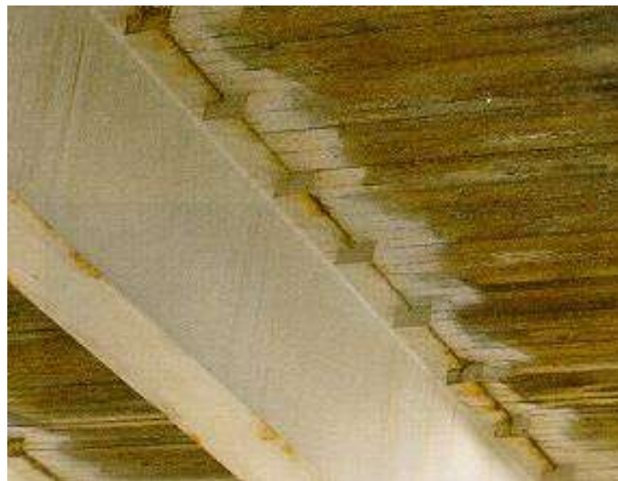
Figure 2.5.15.13 Light Chemical Damage on Underside of a Wood Deck
