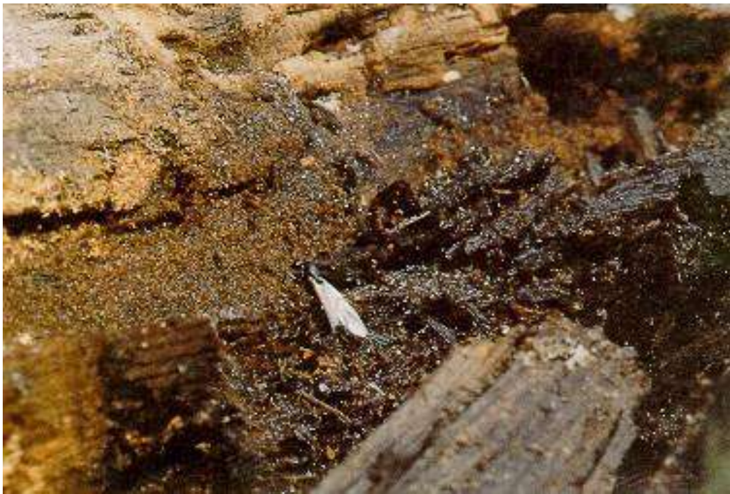
Figure 2.5.15.8 Severe Insect Damage in Wood
