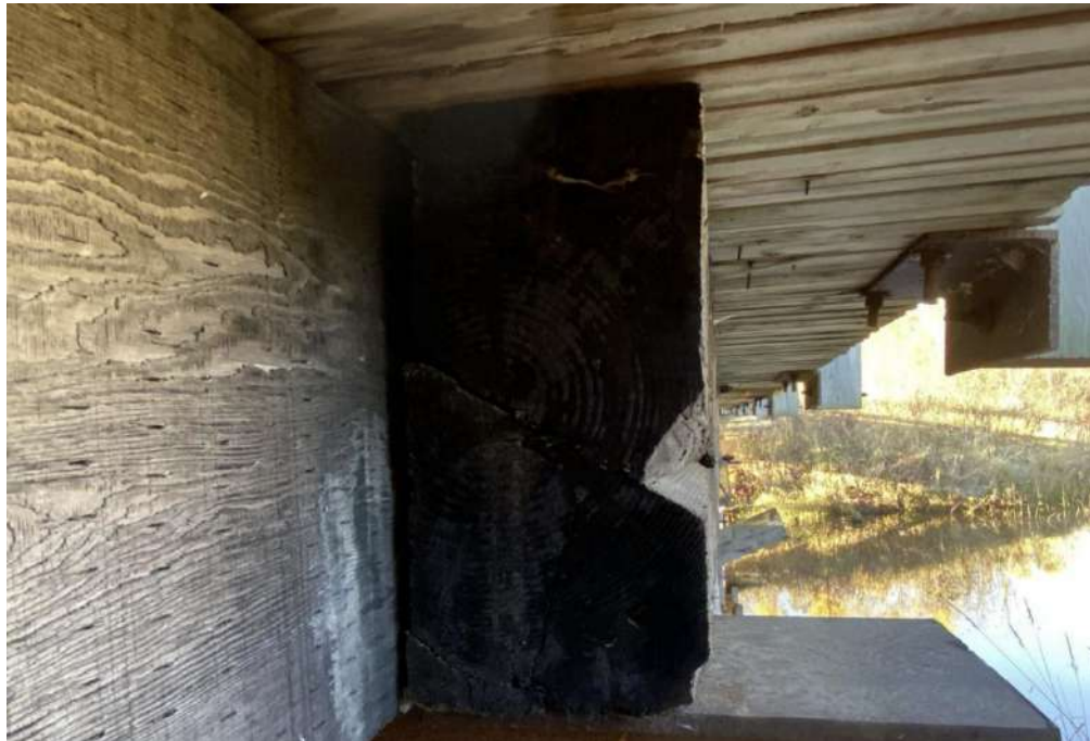
Figure 2.5.15.2 End Check in Wood Beam
