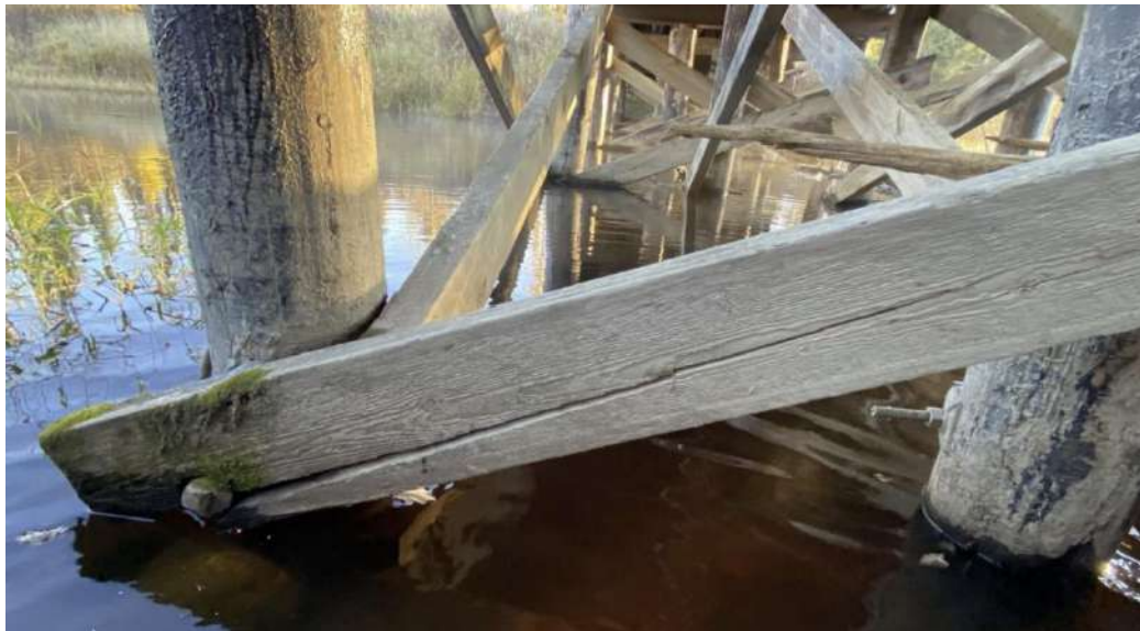
Figure 2.5.15.4 Severe Split in Wood Bracing
