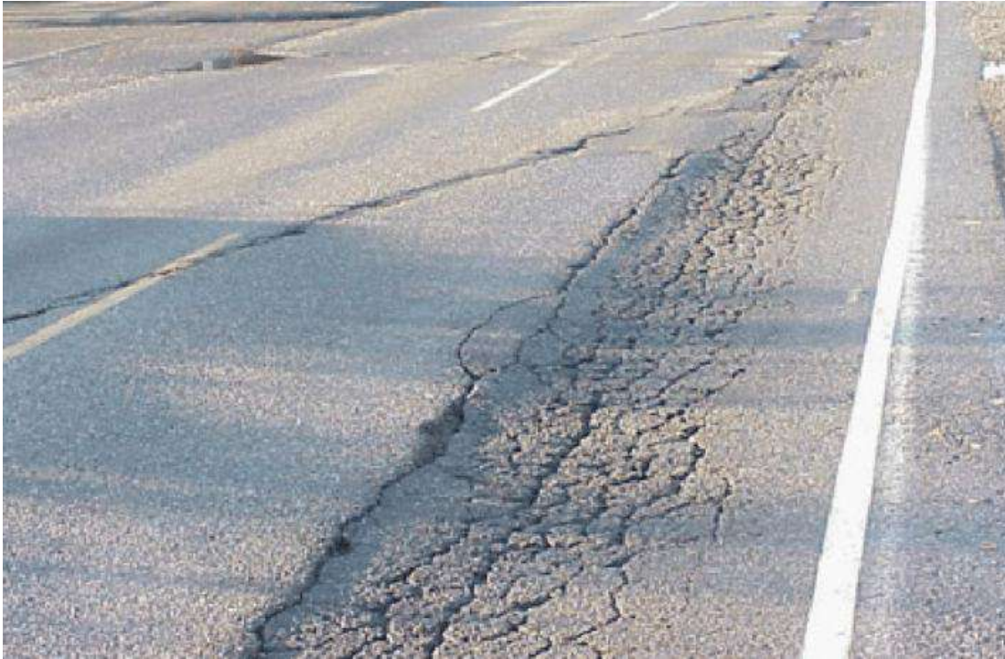
Figure 2.5.8.10 Severe Wheel Track Rutting
