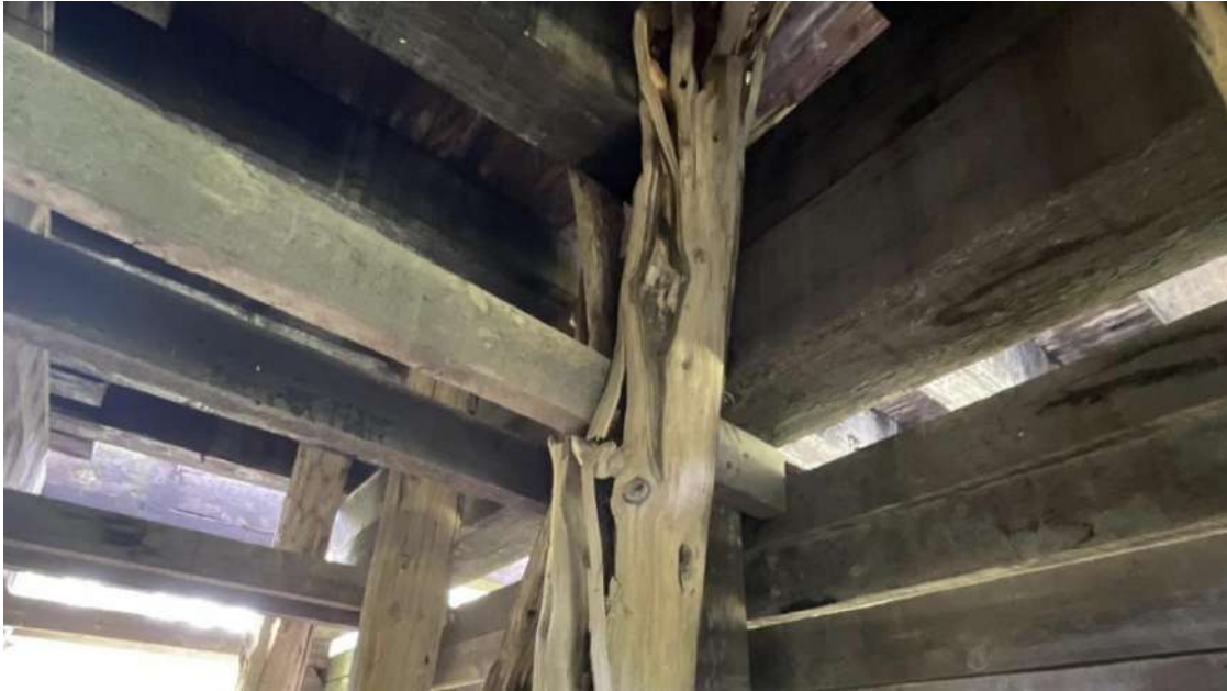
Figure 2.5.15.11 Severe Splitting of Wood Pier
