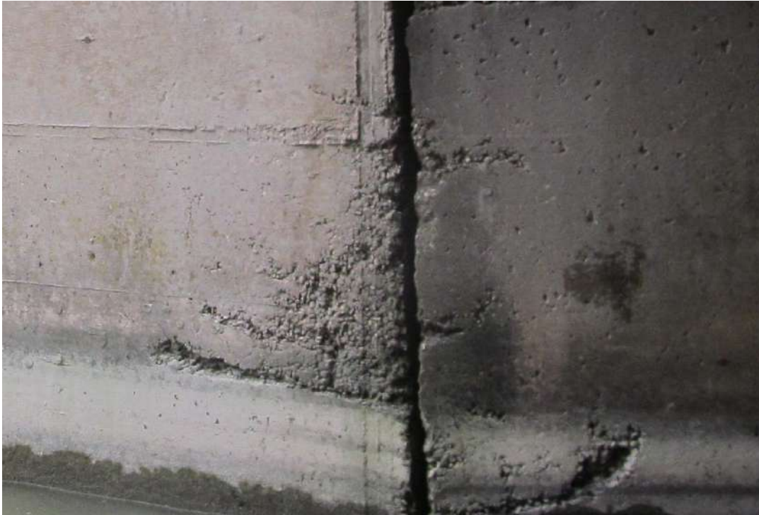
Figure 2.5.4.16 Severe Honeycombing on an Abutment and Wingwall
