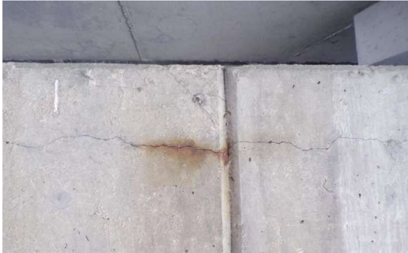
Figure 2.5.4.13 Medium Crack due to Corrosion of Reinforcement
