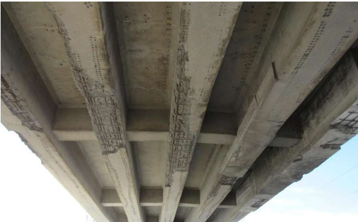
Figure 2.5.4.6 Severe Spalling and Delamination in Concrete Beams
