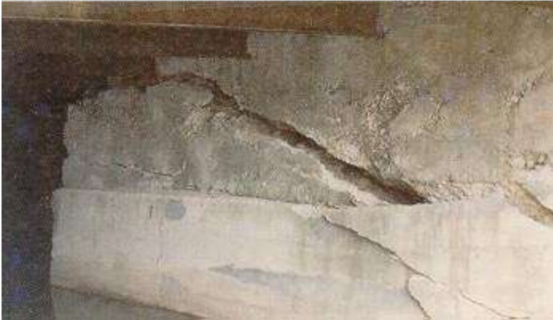
Figure 2.5.4.12 Very Wide Movement Crack in an Abutment
