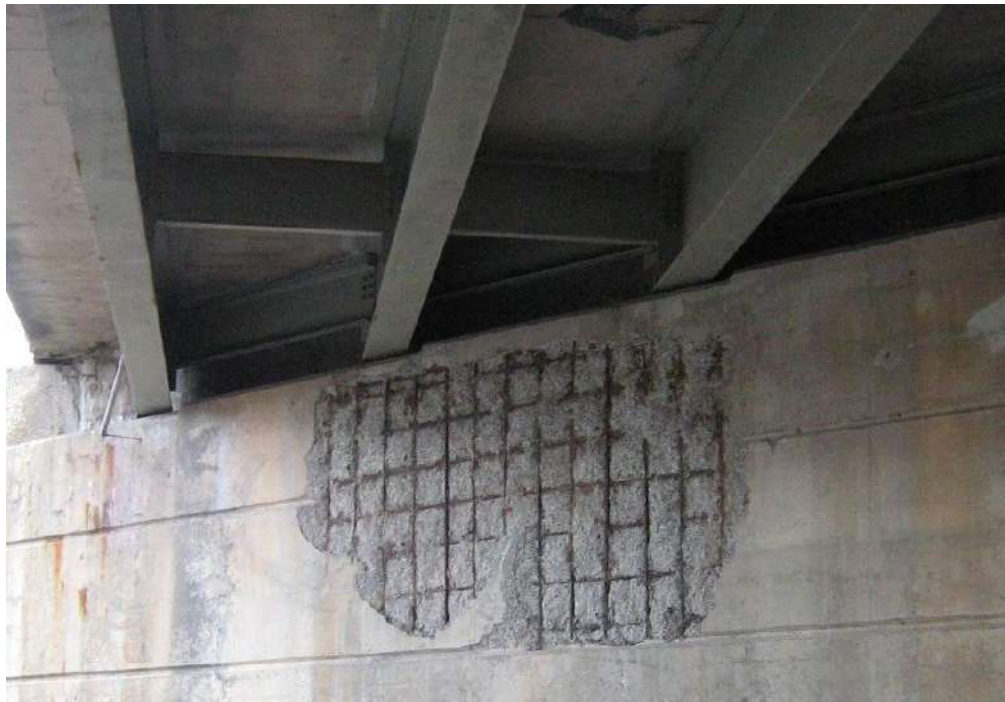
Figure 2.5.4.7 Severe Spalling in Concrete Due to Corrosion of Reinforcement
