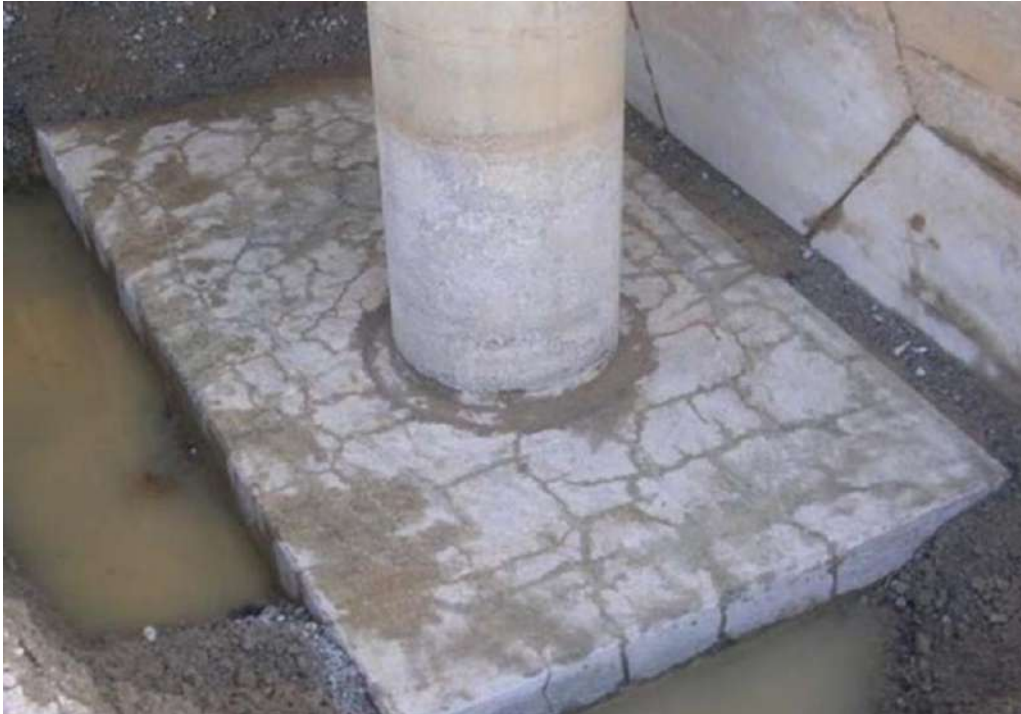
Figure 2.5.4.15 DEF Pattern Cracks in Pier Footing
