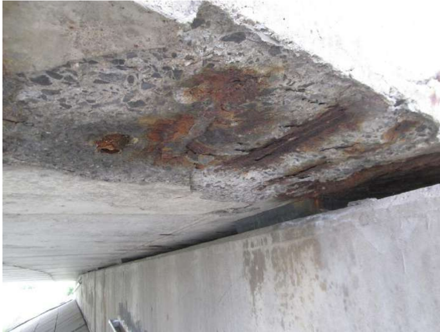
Figure 2.5.4.8 Severe Local Spalling
