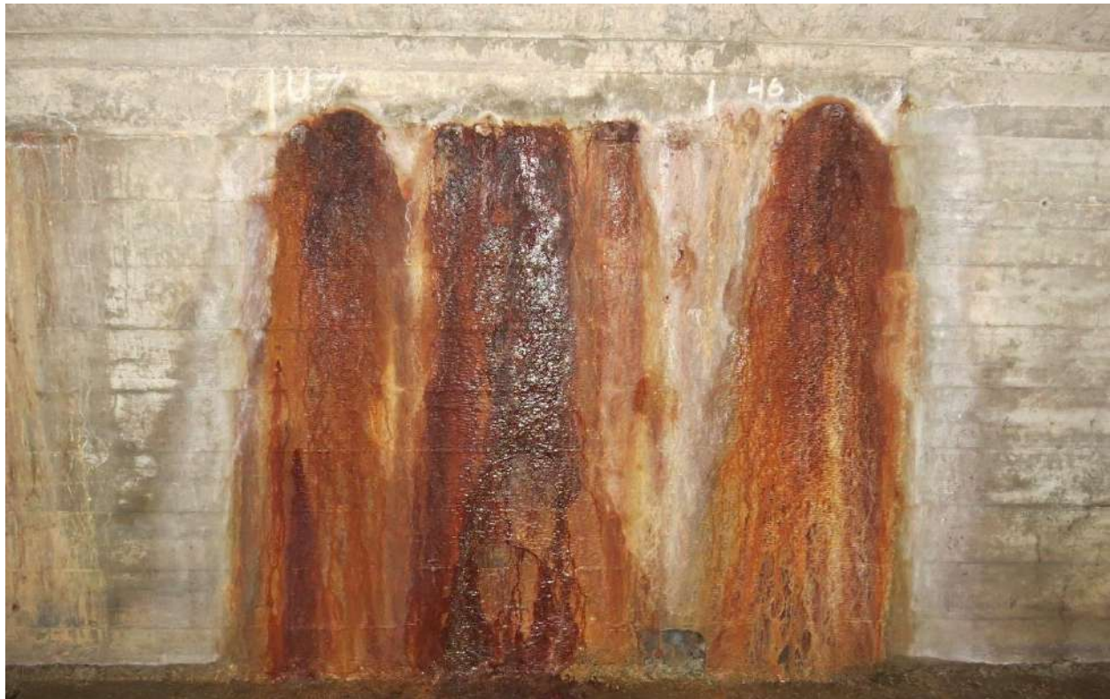
Figure 2.5.4.5 Stains on Concrete Surface Indicating Corrosion of Reinforcement
