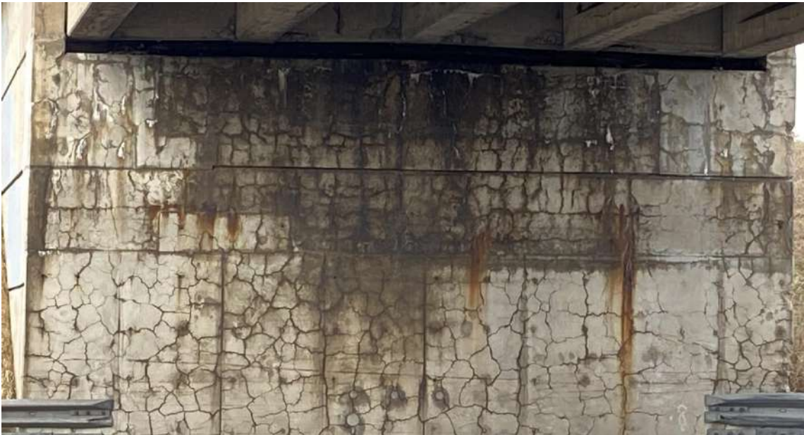
Figure 2.5.4.11 Pattern Cracks in Abutment
