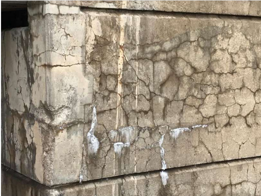
Figure 2.5.4.14 Severe Alkali-Aggregate Reaction
