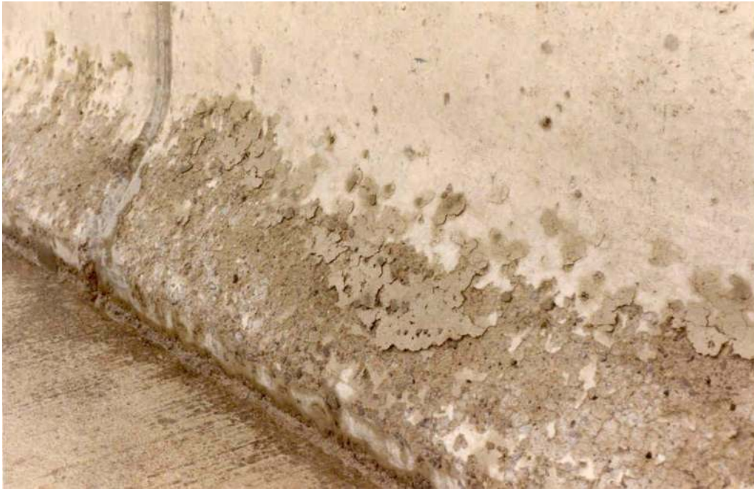
FIGURE 5 Example of Severe Scaling
