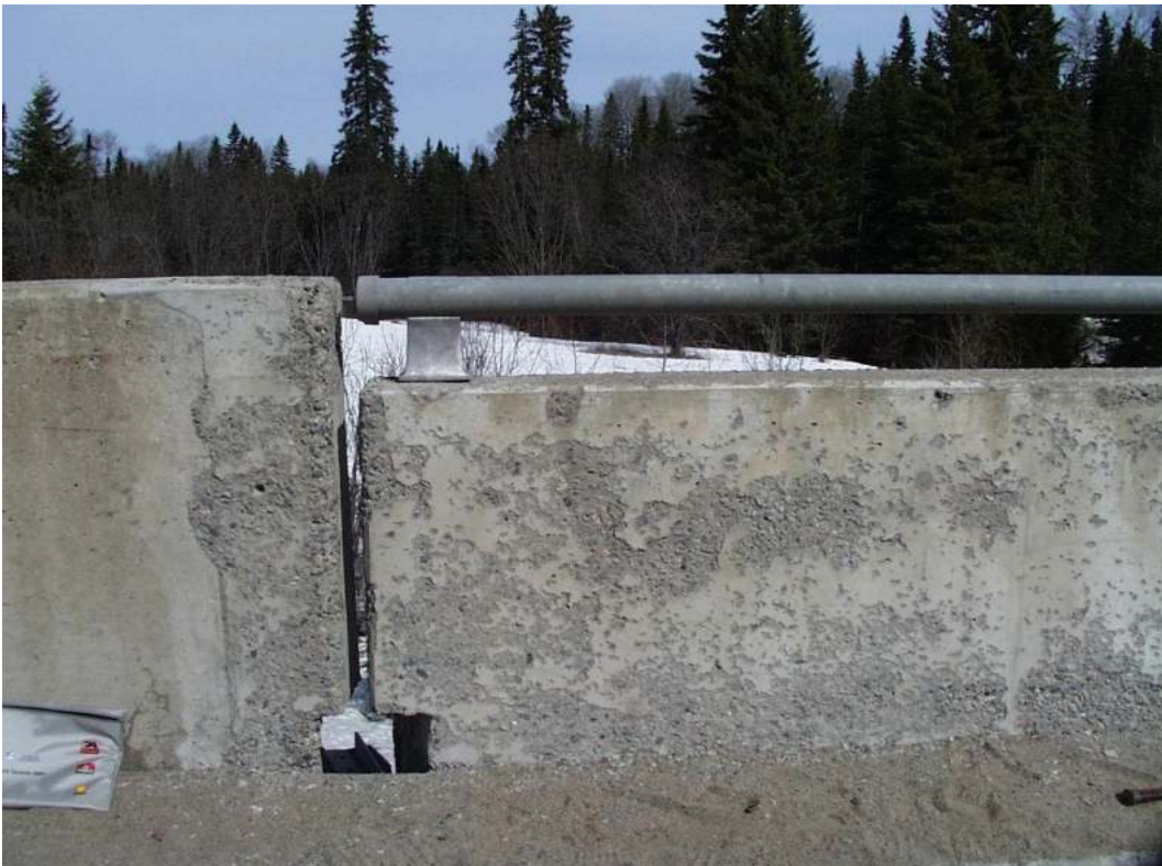
FIGURE 6 Example of Severe Scaling
