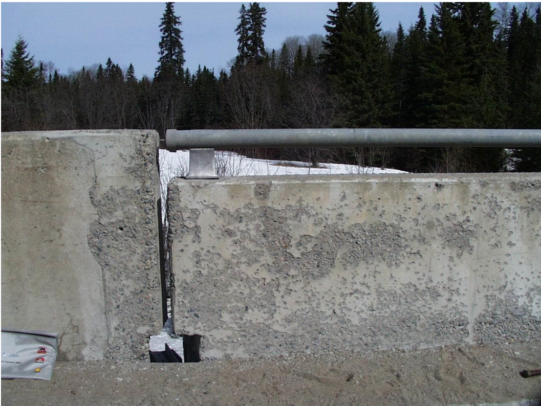
FIGURE 6 Example of Severe Scaling
