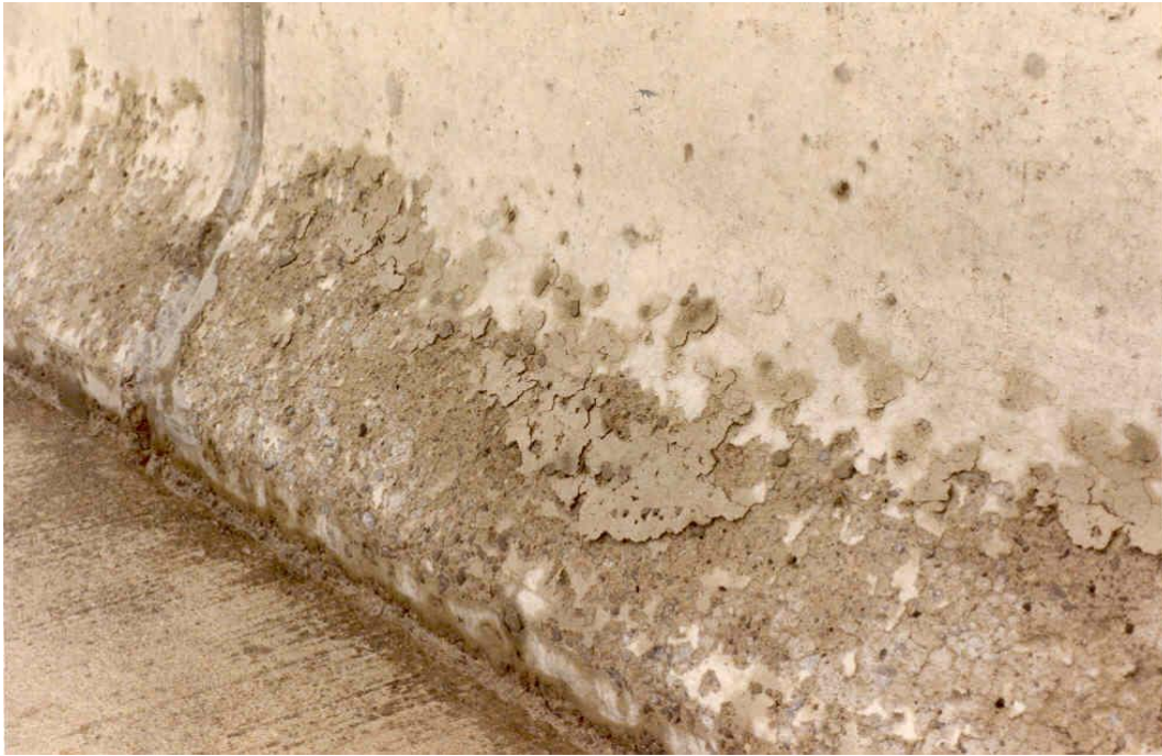
FIGURE 5 Example of Severe Scaling
