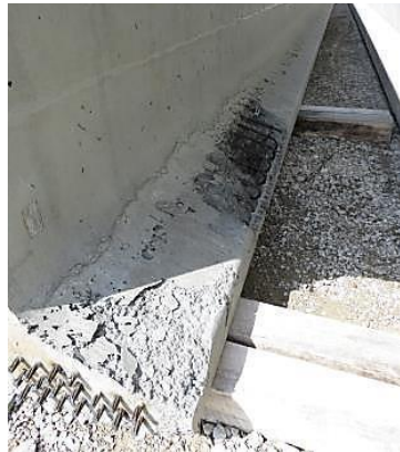
Figure 53 – NU Girder Voids
