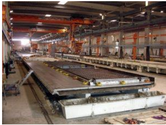
Figure 25 – Precast Plant Interior
