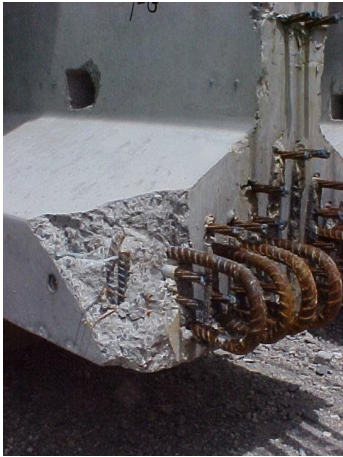
Figure 55 – Bottom Flange Spall
