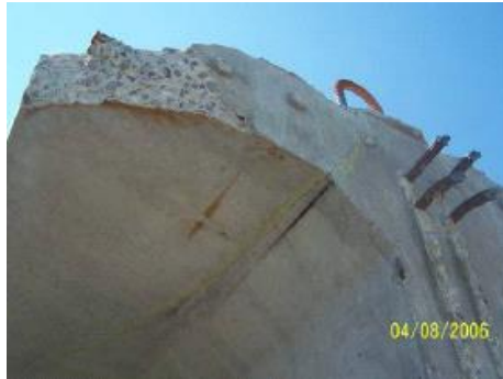
Figure 56 – Top Flange Spall
