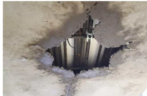
Figure 54 – Box Girder Soffit Void
