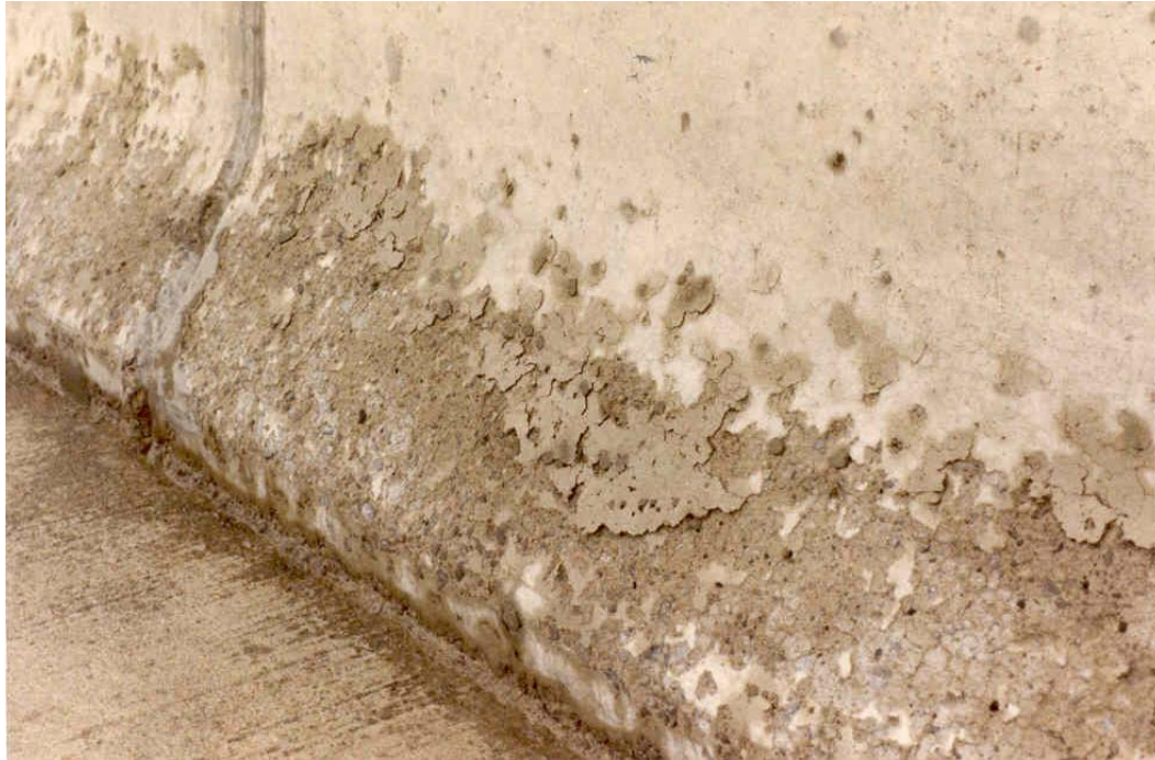
FIGURE 5 Example of Severe Scaling
