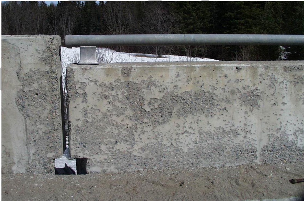
FIGURE 6 Example of Severe Scaling
