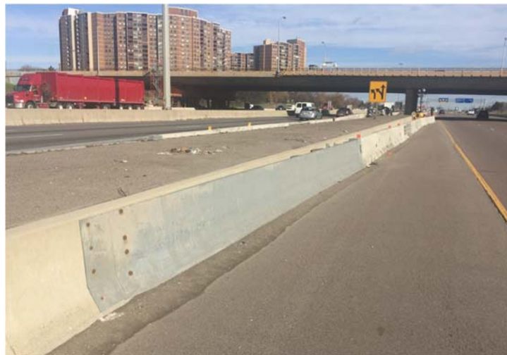
Figure 5-2027: Transition from Permanent Concrete Barrier to Temporary Concrete Barrier Photo courtesy of Powell Construction and TTI.
