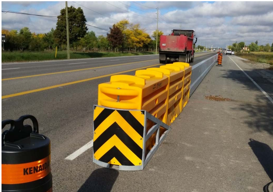
Figure 5-25: SLED Temporary Reduced Exposure Energy Attenuator
