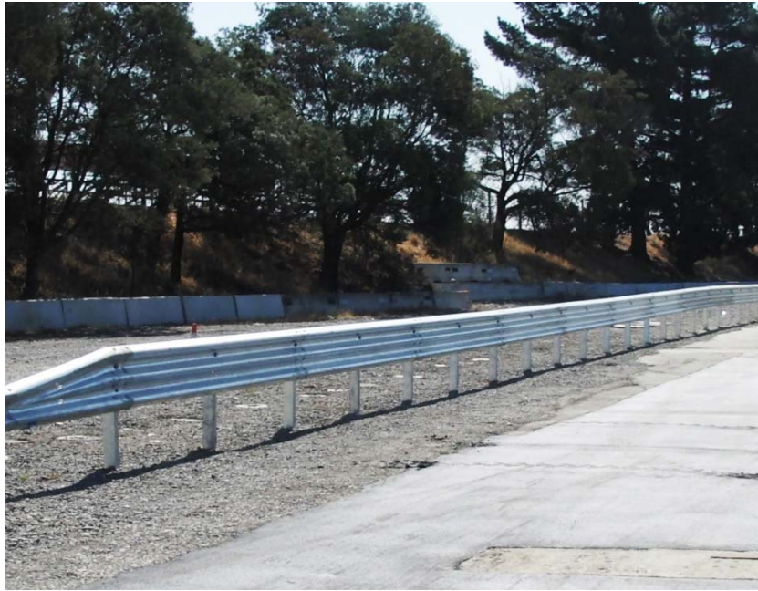
Figure 4-17: ACP TL-4 Barrier
