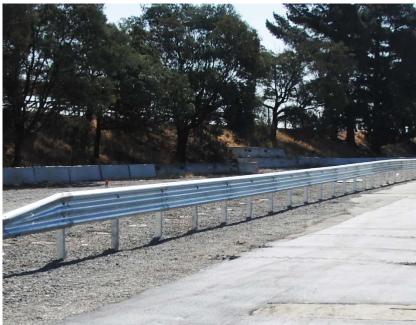
Figure 4-17: ACP TL-4 Barrier
