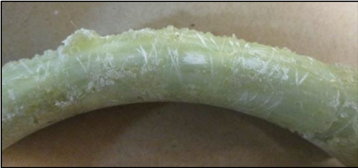
Figure 93 – Visible fibres (may be repaired by the manufacturer)
