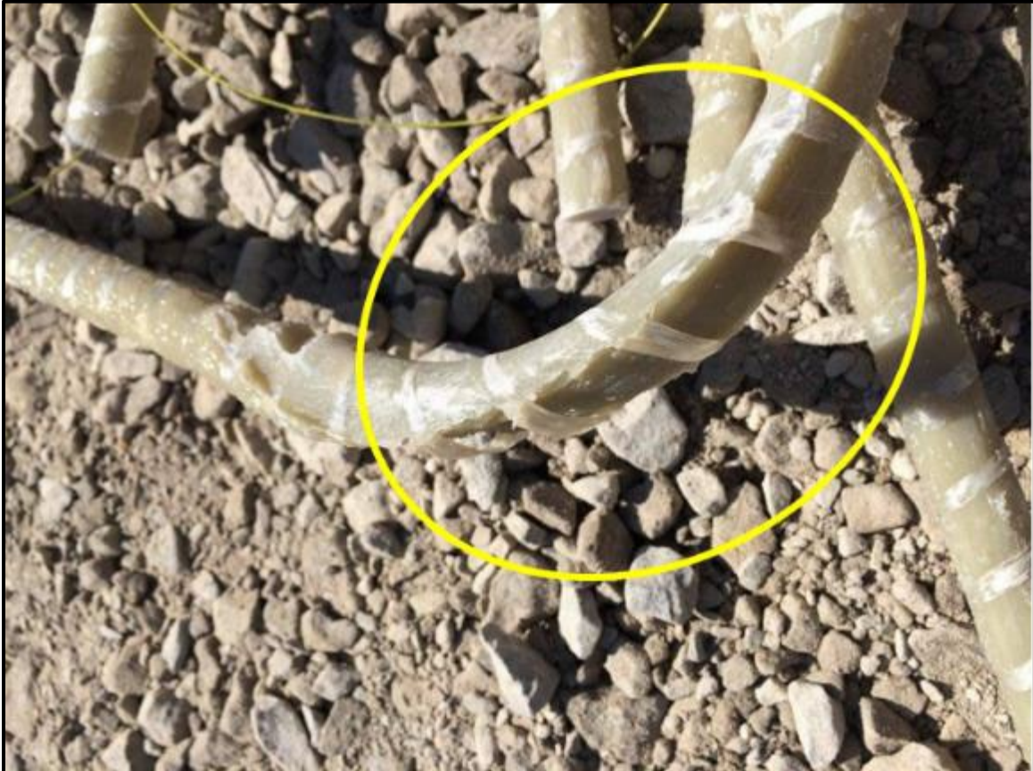
Figure 111 – Unacceptable bar with crevices and section loss at bend
