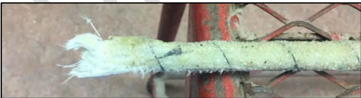
Figure 107 – Loose / frayed fibres at bar end
