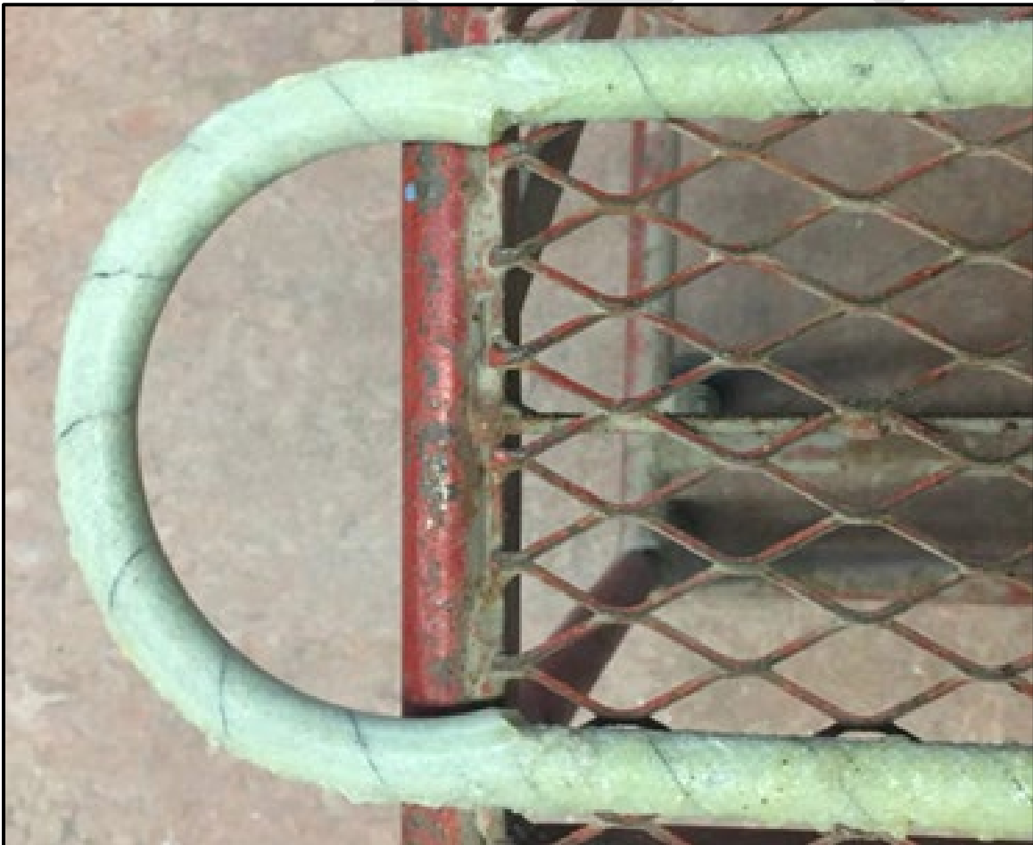
Figure 104 – Deformity at the start/end of bend
