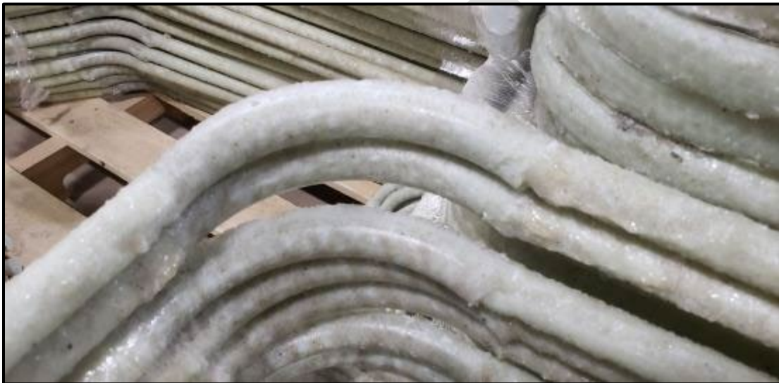
Figure 31 – Inside of bend loss of sand coating
