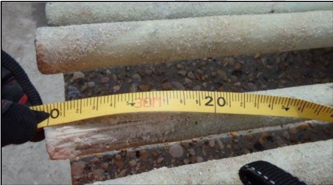
Figure 71 – Sand and resin loss and exposed fibres
