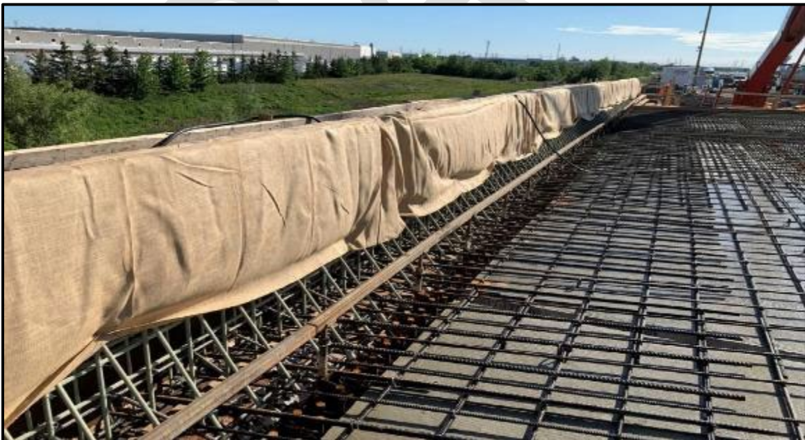
Figure 91 – Installed bars with improper and incomplete coverage
