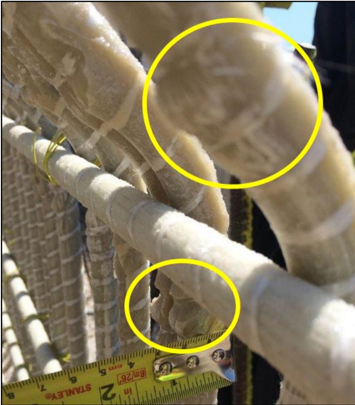
Figure 110 – Unacceptable bar, showing bulges on the inside of their bends
