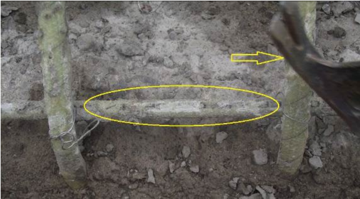
Figure 84 – Hammer strike damage to bars (arrow pointing to hammer)
