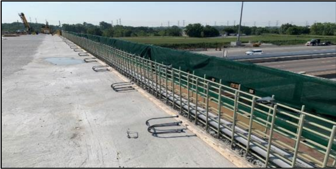
Figure 92 – Installed bars not covered with polyethylene
