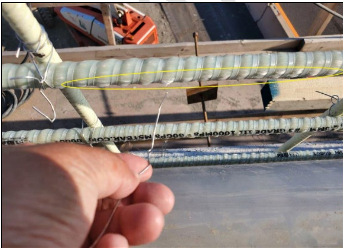
Figure 66 – Exposed, dry fibres
