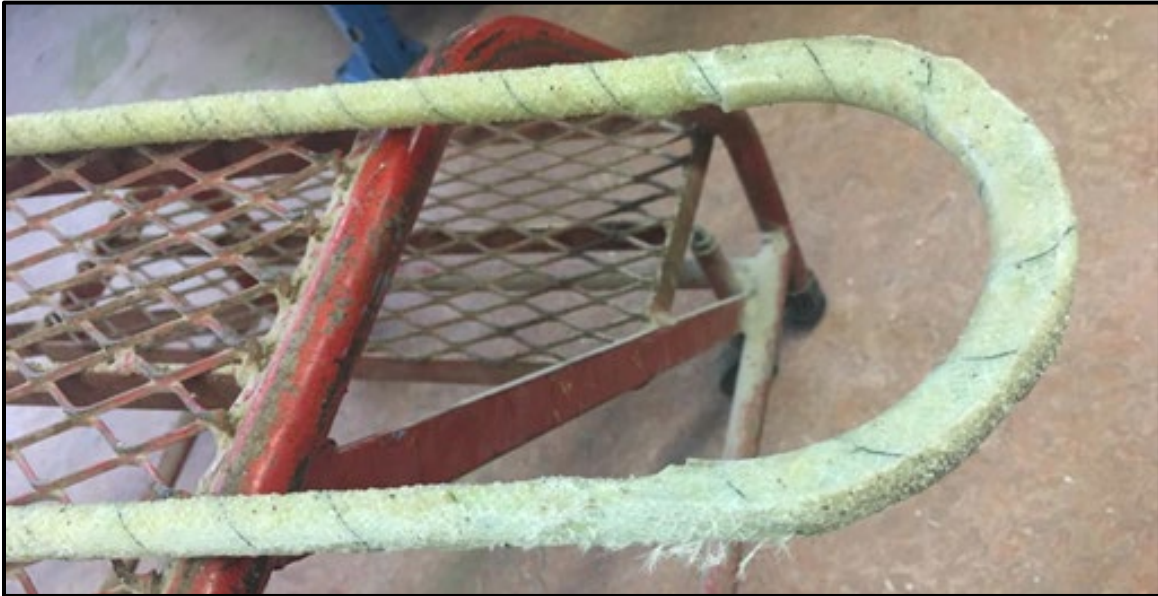
Figure 108 – Exposed fibres at bend
