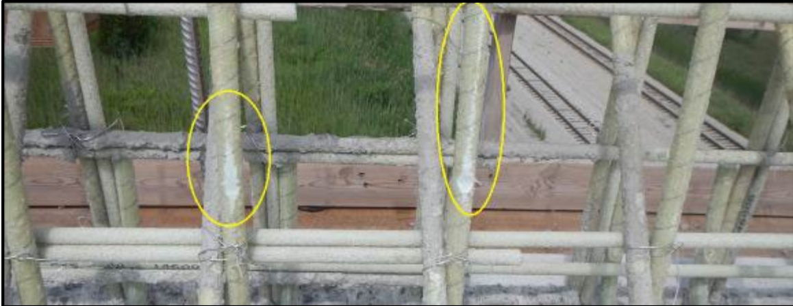
Figure 82 – Damage from bar rubbing
