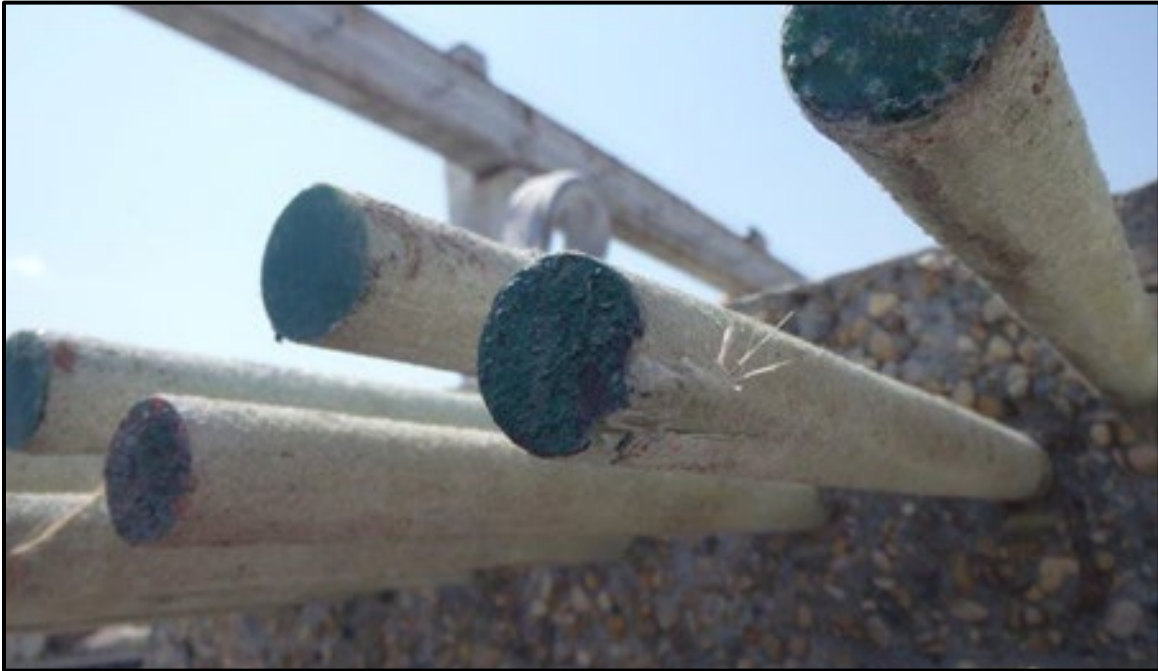
Figure 72 – Sand and resin loss and exposed fibres
