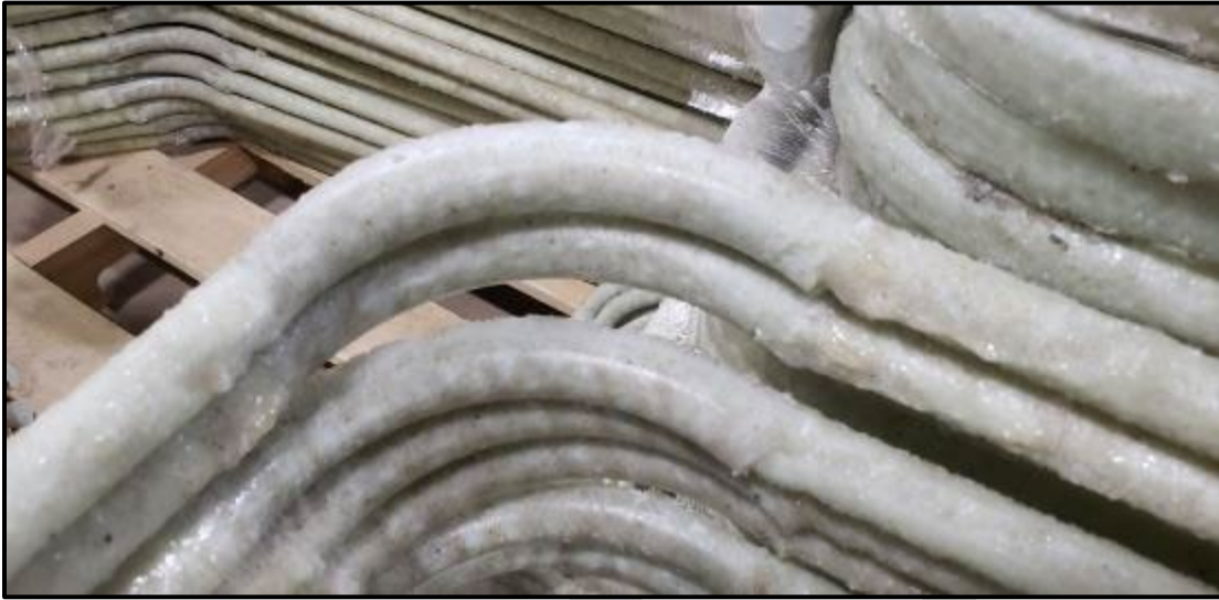
Figure 21 – Inside of bend
